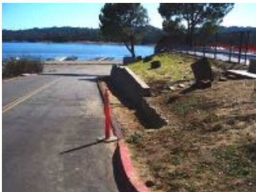
New Sidewalk to Marina Parking Lot Built by Volunteers Ready for Concrete Pour
